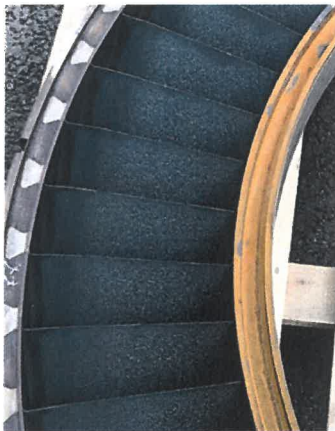
GT1, 4th stage vane, pressure side On- and off-line cleaned with Cleaner A
